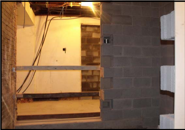
Looking from the back of the elevator to the front of the elevator at the old Bell Tower entrance.
