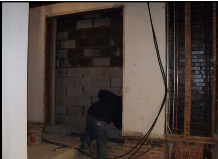
Looking from the new Fellowship Hall entrance to the old Bell Tower entrance.
